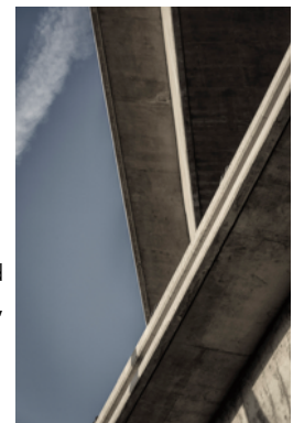
The 2 Freeway overpass, Montrose, California. An urban detail that may be there for years or disappears tomorrow. Who knows?
